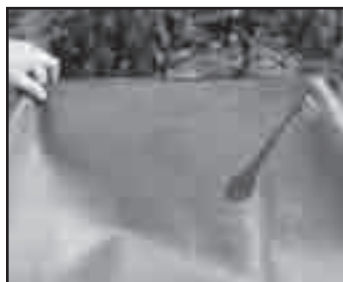
Fig. 33 Poke holes in the liner all the way through to the inside of the filter box.
