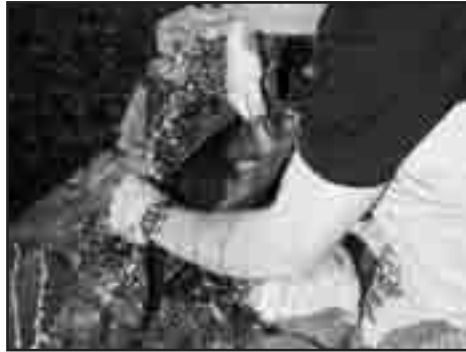
Fig. 46 If you find the leak, pack soil beneath the liner to raise the edge.
